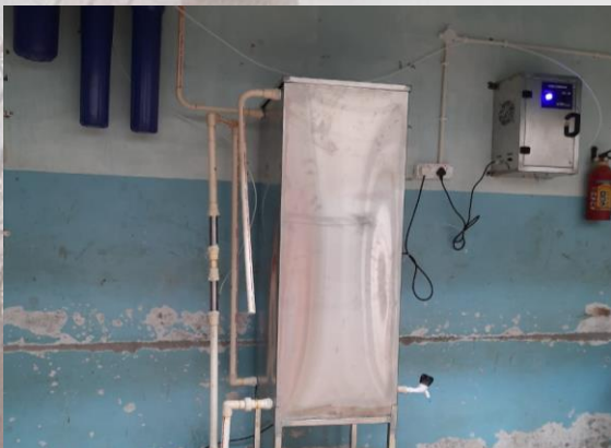
Two safe water systems were installed in the state of Karnataka, in September: One at a child care institute and the other at an institute for the mentally challenged.
